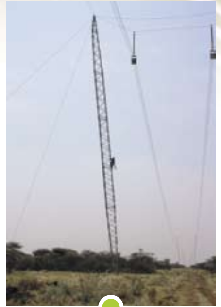
A NamPower construction worker scales one of the 42 m high towers to check on the tension of the newly-installed electricity conductor cable.
